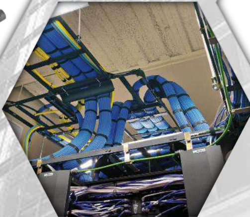
Cabling and Cable Management
