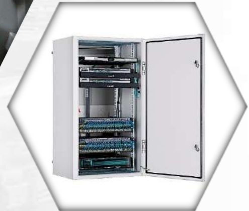
Industrial Distribution Frame
